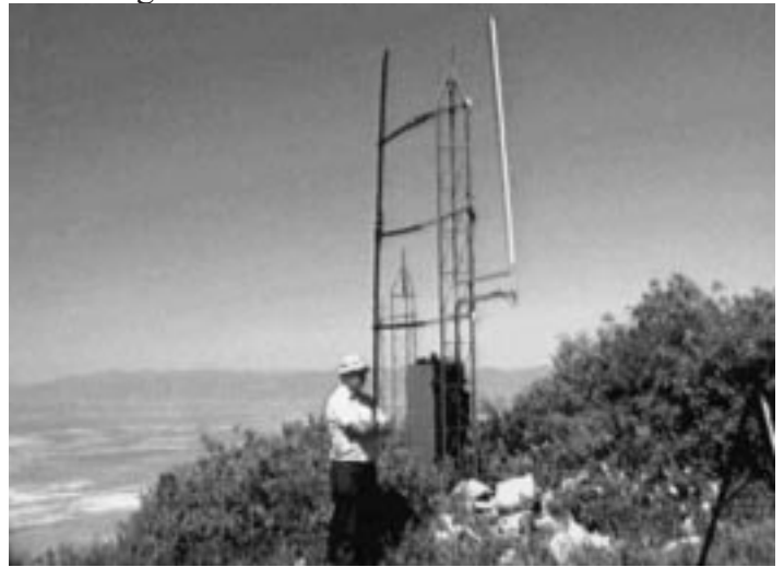
Shown here is the receive site, its tower, and antennas. The black antenna on the left is the main receive antenna. It is placed on the tower to provide a null toward the transmitter site to reduce the possibility of interference from the transmitter site. The white antenna is the spare antenna, to be used should the main antenna become damaged or fail.
