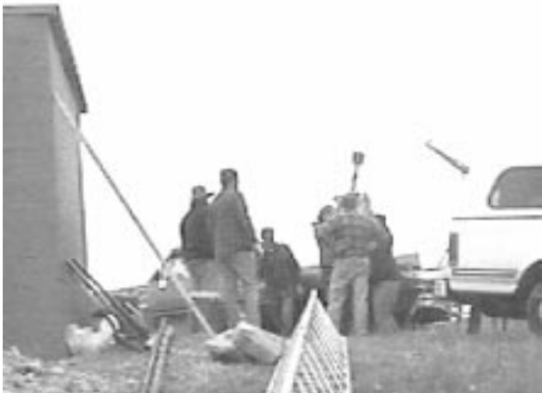
Using the rod driver the crew attempts to get the second ground rod driven deeper than the first
