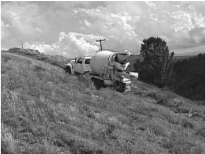
The long awaited cement truck grinds up the final grade after giving the author a wild ride.
