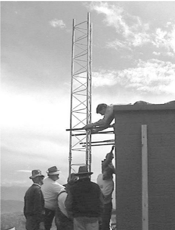
Gary, KK7DV, lying on the roof adjusts the U-Bolts as the tower is maneuvered into place
