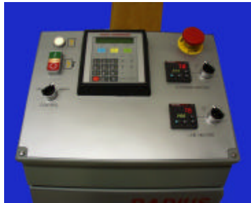
Enclosure control panel for operator interface in "Stand Alone" mode
